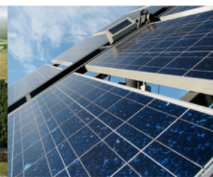
Solar photovoltaic power plant
